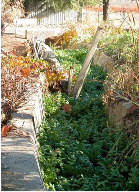
Figure 1. Creep of the San Andreas Fault at the Cienega Winery (now the de Rose Winery) south of Hollister, California, has cut through the winery structure, and since 1956 has cracked and offset a culvert there by more than 3 feet.
